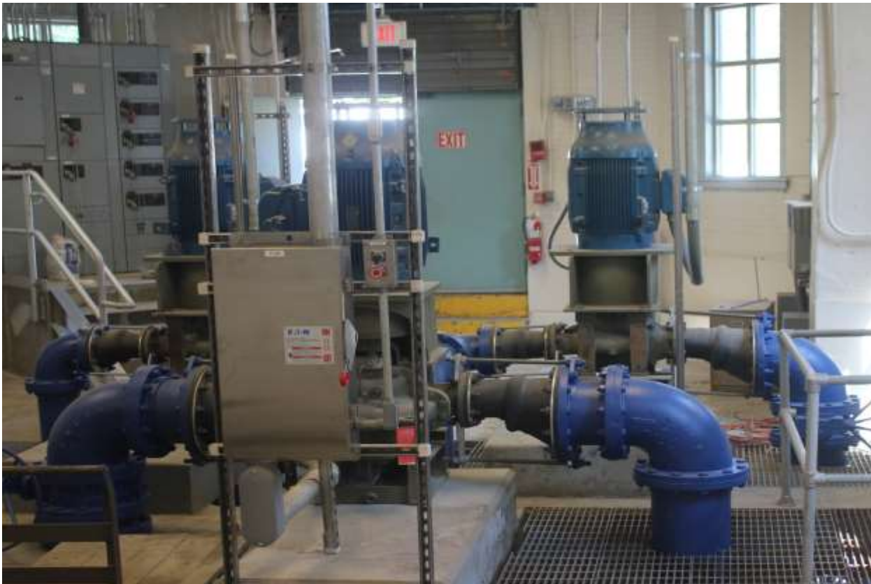
Bridge Street Treatment Plant finished Water Pump Room
