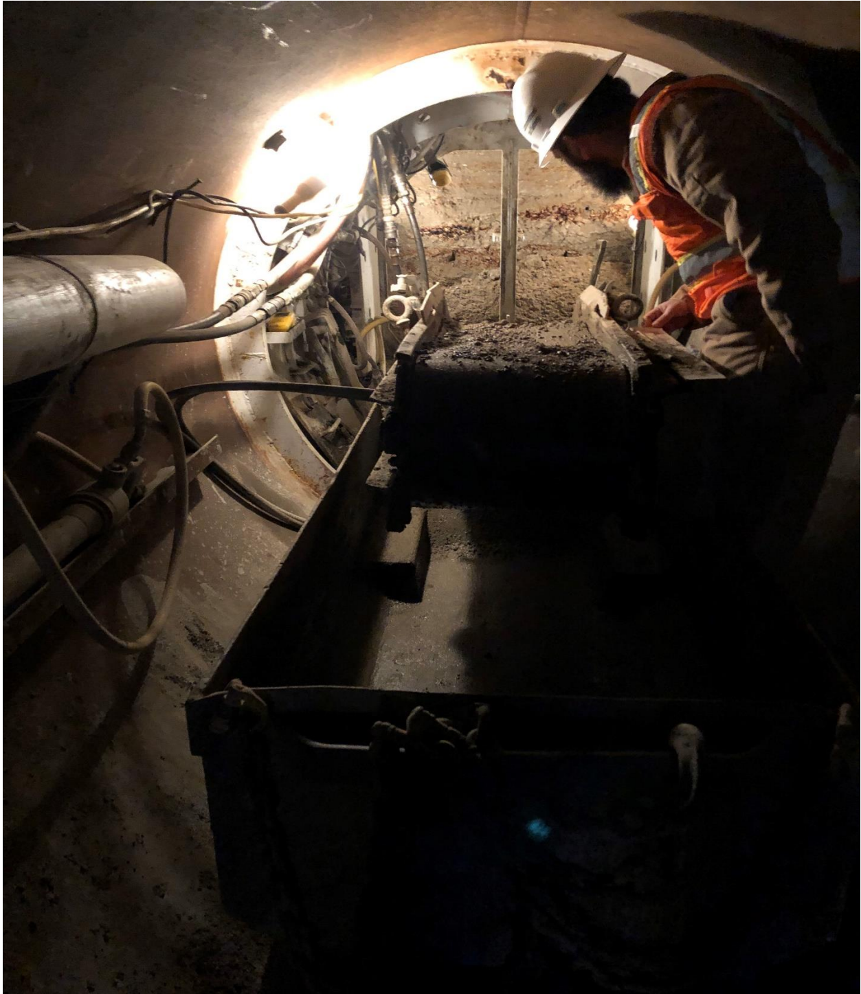
Worker at open face of jacking pit showing soil, conveyor ramp, and cart for hauling spoils out of tunnel.
