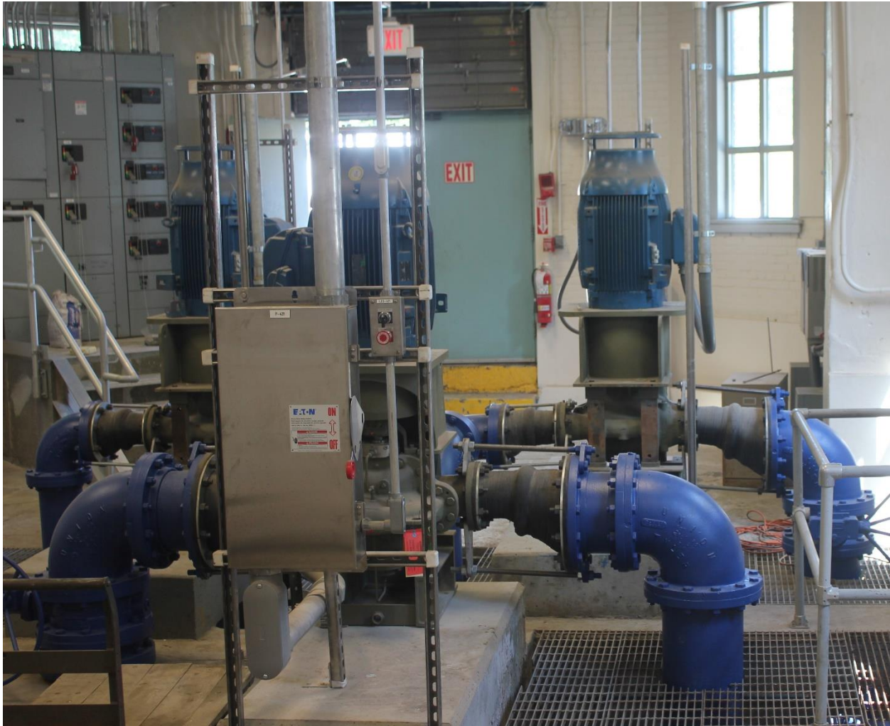
New Finished Water Pumps installed as part of the Modernization Project.
