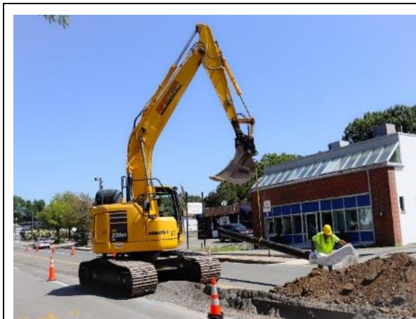
Photo of an excavator installing new ductile-iron water main pipe on Washington Street in Westwood.
