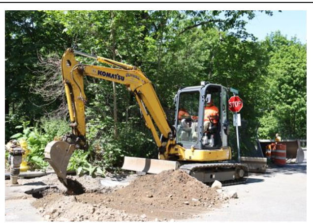
Photo of an excavator backfilling a water service line connection on Veterans Road in Dedham.
