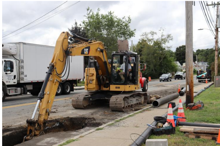
Image of an excavator digging on East Street in Dedham to install new water main pipe.
