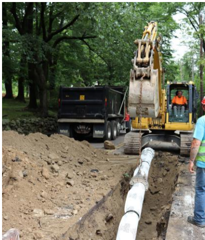
Image of an excavator installing new water main pipe on Milk Street in Westwood.
